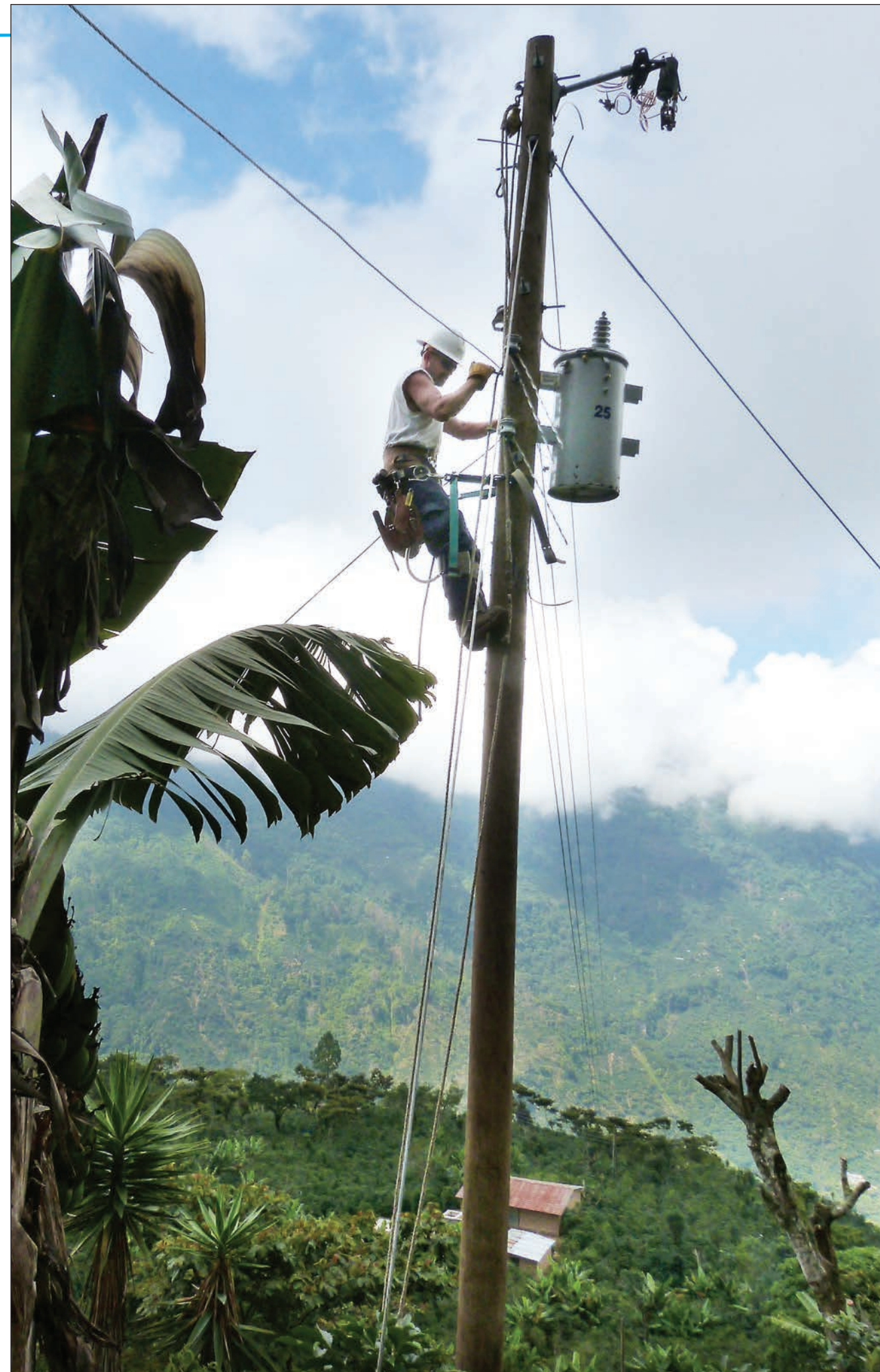
Chad Griffin, a lineman from South Central Indiana REMC, connects a transformer to a new pole for a village in the Cuchumatanes Mountains of Guatemala. Unlike working in the rolling farmland of home, Hoosier linemen here would climb 30 feet up one side of a pole, and be able to look straight down a 1,000 foot gorge on the other side.
