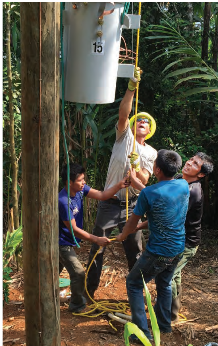
Pat Scheurich, of Jasper County REMC, gets some assistance from local men hoisting a transformer to the top of a pole. The Indiana linemen said the villagers' work ethic, pride and commitment amazed them.
